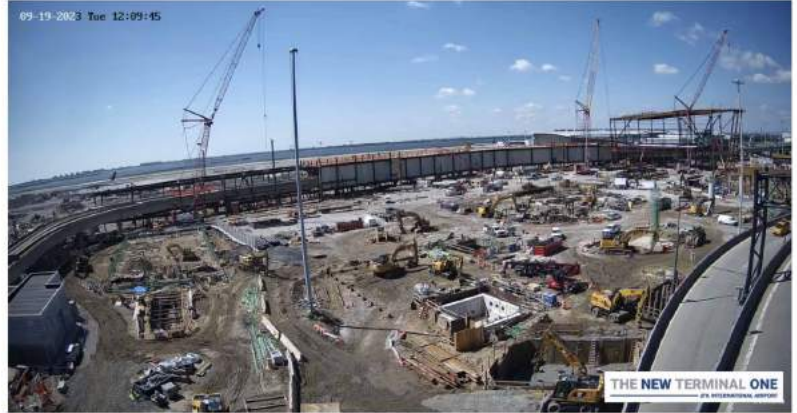
Time lapse video of the construction site between September 19 th through October 27 th .
